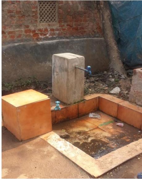
Community water tap by BMC in Shantipalli
