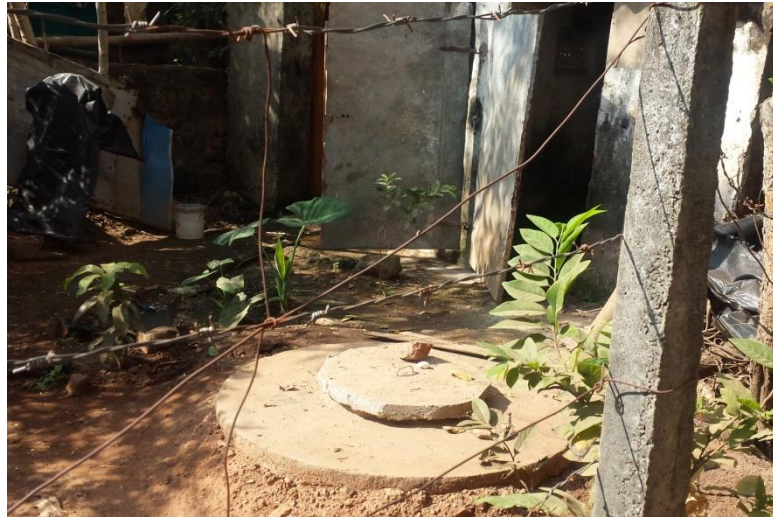
Toilet with soak pit Refugee colony , Bhubaneswar
