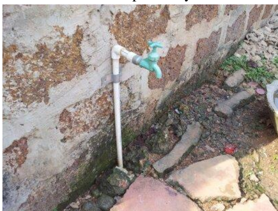
Individual water connection in Shastrinagar
